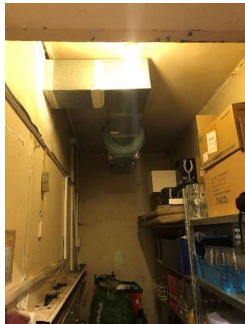
Photo 6: Club bar vent
