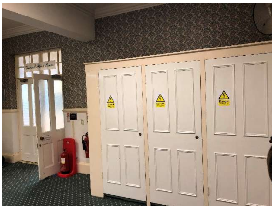
Photo 8: Main Electrical Switchgear
