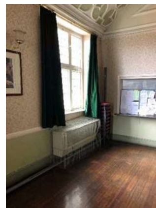
Photo 4: Convector + exposed gas pipework
