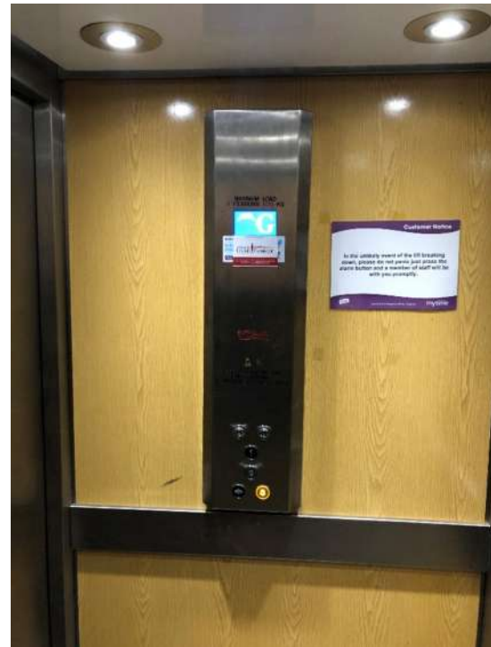
Photo 15: Lift control panel
