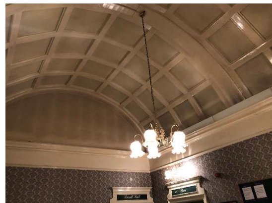
Photo 13: Central stairway lighting
