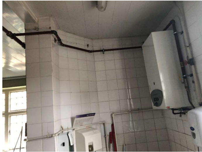
Photo 7: Community hall kitchen gas fired water heater
