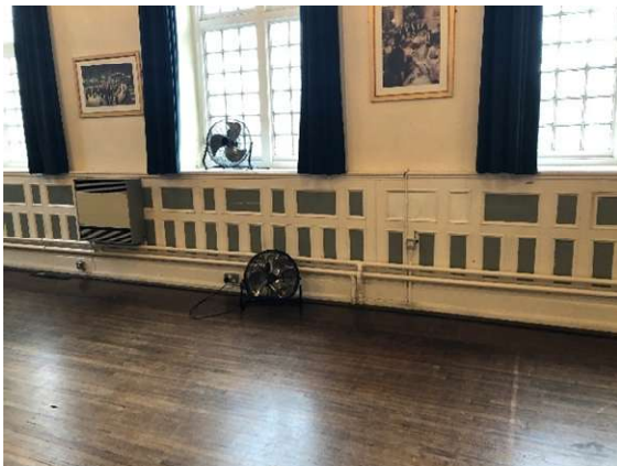
Photo 3: Boiler fed fan convector + pipework
