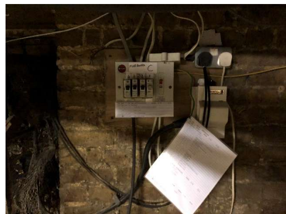
Photo 9: Electrical Distribution Equipment
