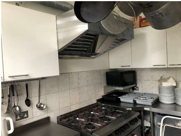
Photo 5: Club kitchen vent
